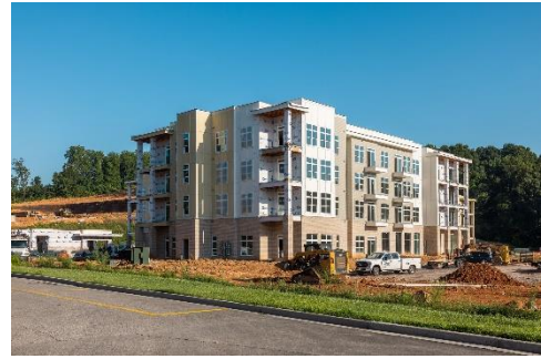
Loft Apartments under construction within Dalton's medical district creating opportunities for workforce housing in this district which includes the Hamilton Medical Center hospital
