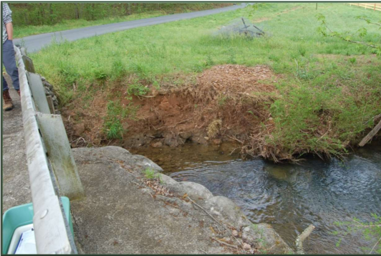
Figure 25. Eroding streambank at Buttrum Road Crossing.
