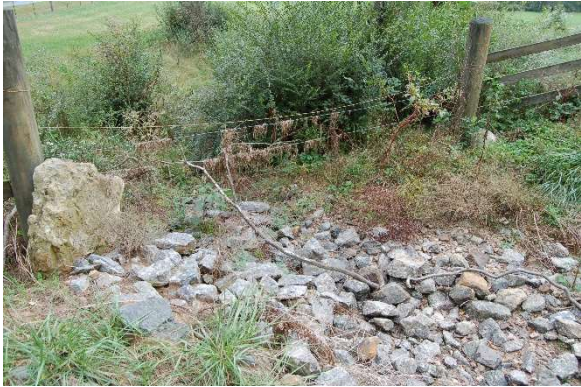
26. Big Oak Tree Road Bridge tributary to Woodward-stream is dry
